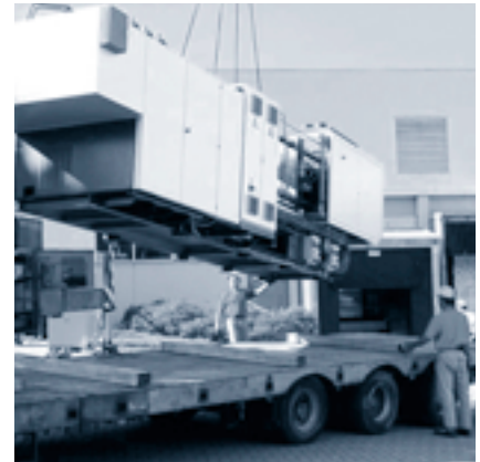
Industrial relocation is one of the services provided by Freudenberg Service Support
