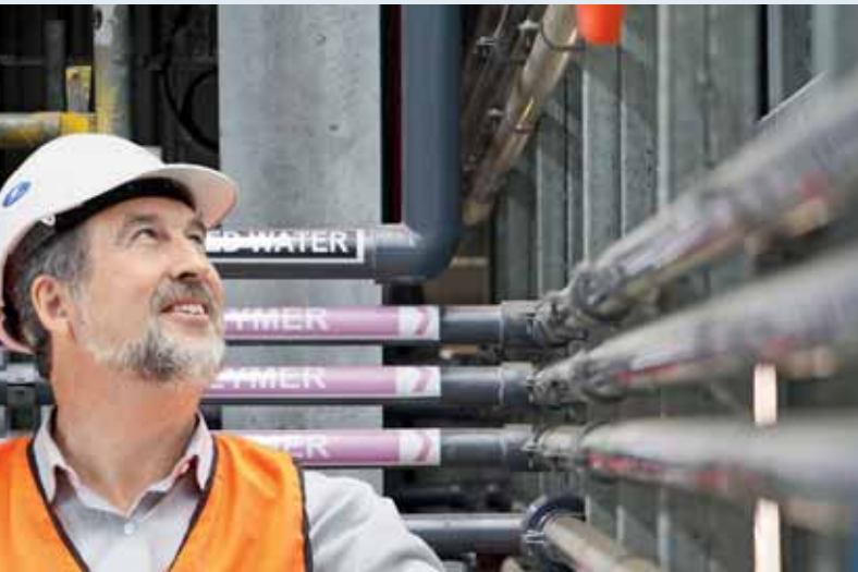
Projects on this scale require perfect cooperation between many partners. Once the water reaches the plant, it is channelled into a number of smaller valve systems and then treated several times over.
