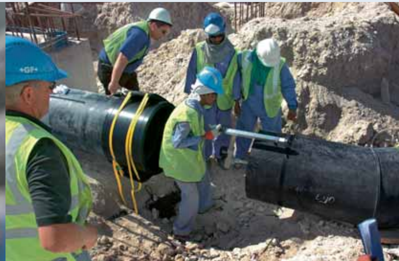
Large-size pipes are used to transport the water to the plant. All in all GF provided six kilometers pipes of varying sizes.
